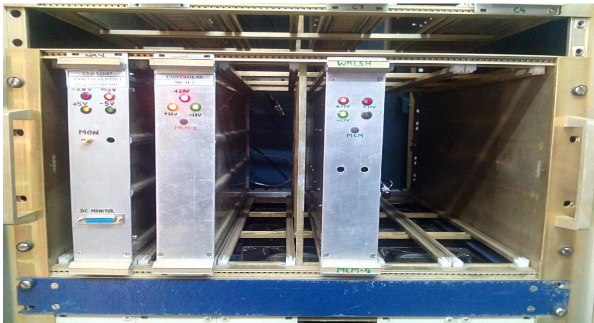
Figure 10: Snapshot of FE & Walsh Control PIU at C10 Antenna
